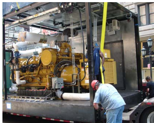
One of two 30-ton engine generator modules that are part of a combined heat and power system installed on the roof of a building on Fifth Ave. in New York City.
