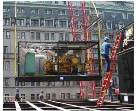
An engine generator module is lifted to the roof of 717 Fifth Ave. in Manhattan as part of the CHP system Northern Power installed there.
