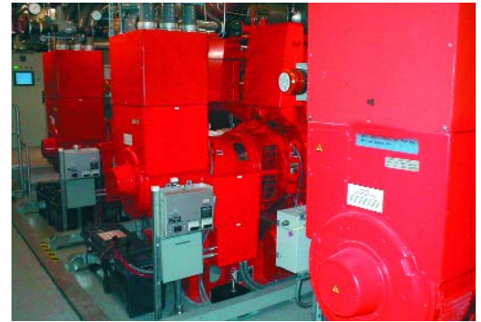
Three 500 kW natural gas-fired generators provide electricity for 1.5 million square feet of office space.
