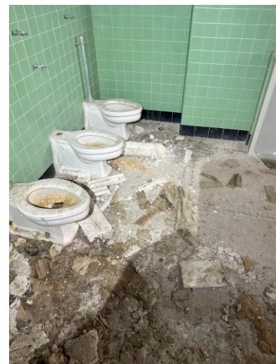
PIPE DEBRIS IN BASEMENT BATHROOM
