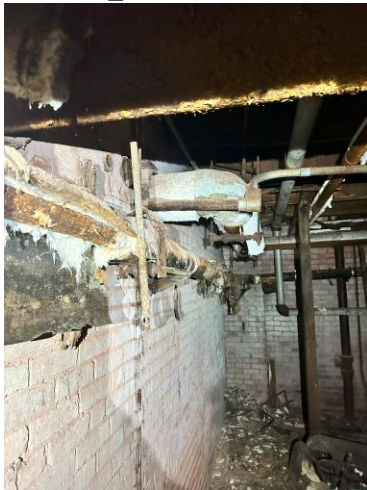
BASEMENT PIPE INSULATION
