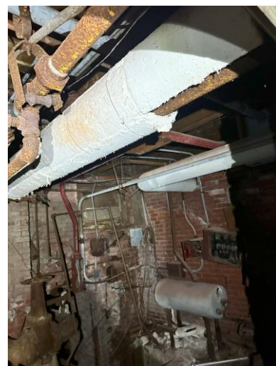
BASEMENT PIPE INSULATION AND DEBRIS
