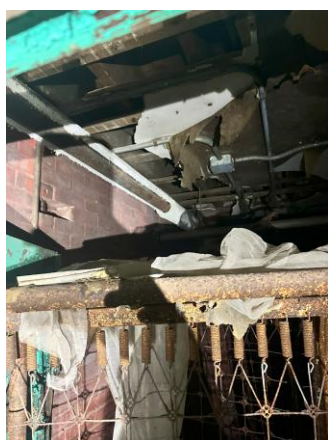
BASEMENT PIPE INSULATION
